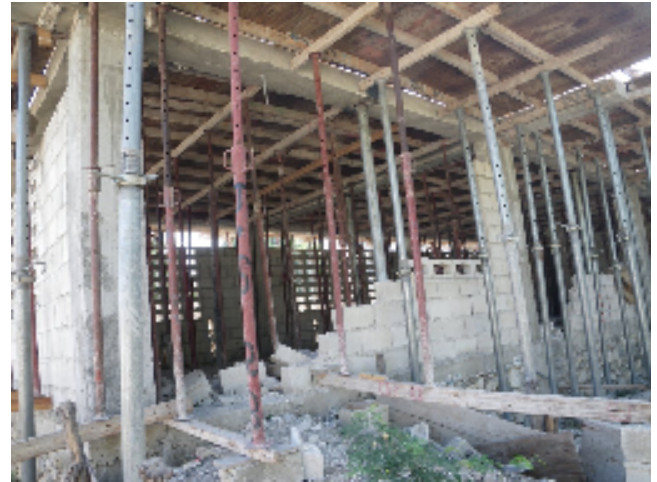
A view of one of the West walls of Patti’s School knocked down by the quake. The walls will be rebuilt to be earthquake resistant.
