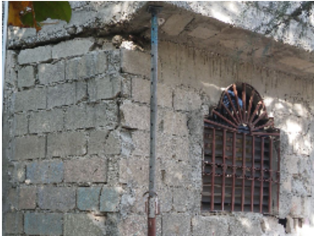
Photo of front corner of House of Hope showing block wall knocked out of place. A number of interior and exterior walls received similar damage.
